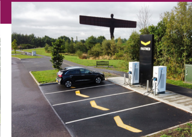
The new EV charge Point next to the Angel of the North on the A167 Durham Road in Gateshead
