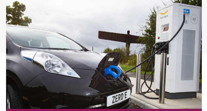
Electric Vehicle charging infrastructure at the Angel of the North in Gateshead
