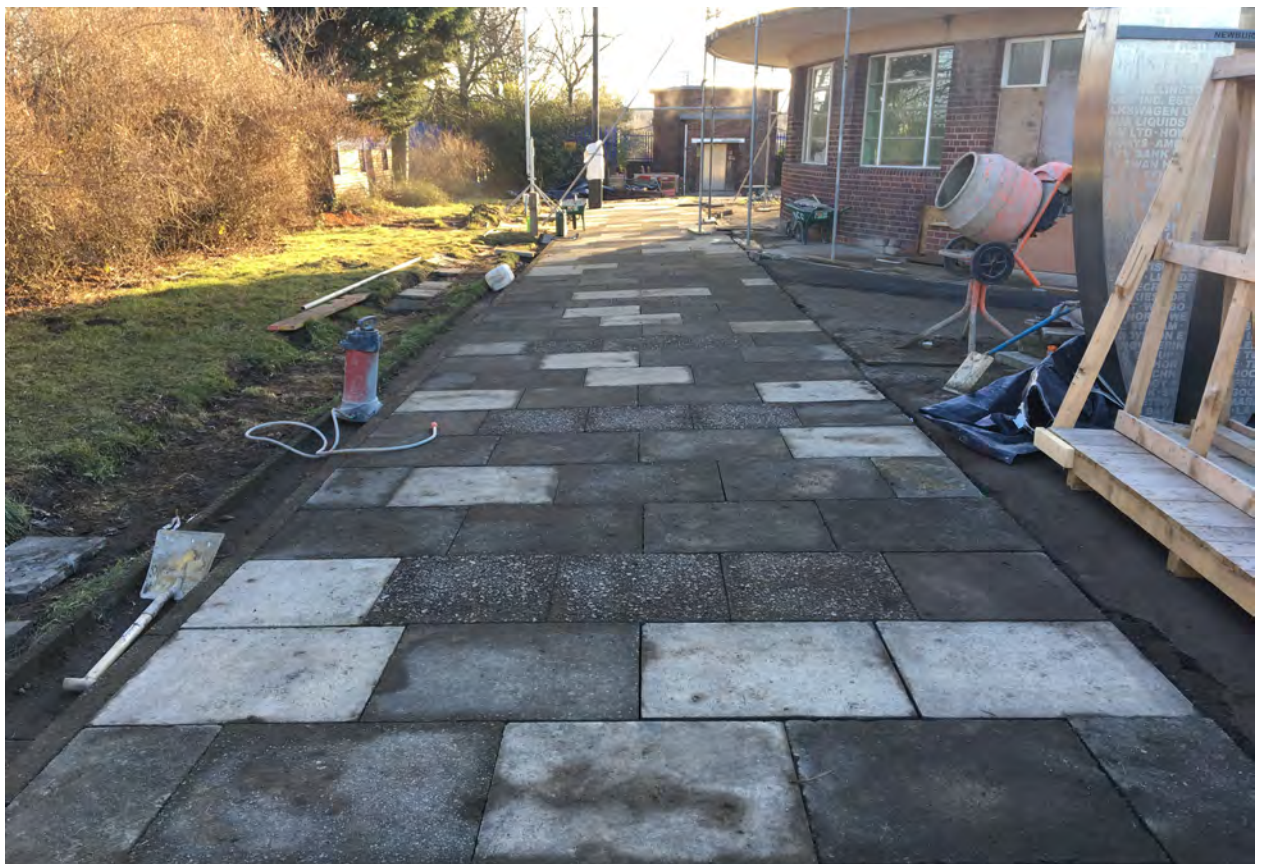
Externally the paving has been relaid providing pedestrian access to the vertical lift.
