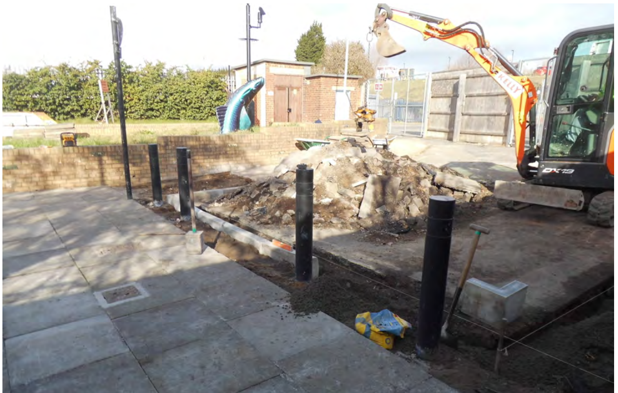
New bollards and drop kerbs have been install to control vehicle access and assist easy access for pedestrians.
