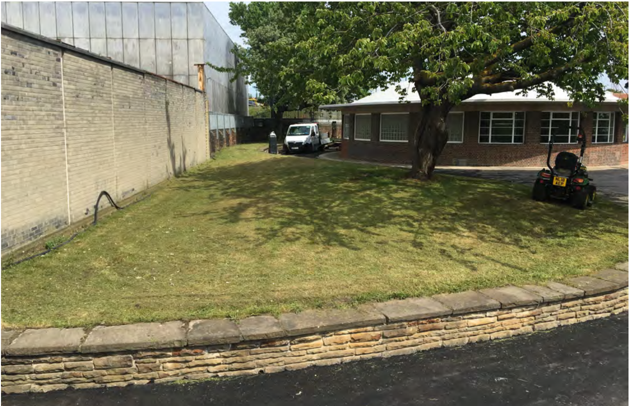
The landscaping and resurfacing works around the Howdon rotunda building have been completed.
