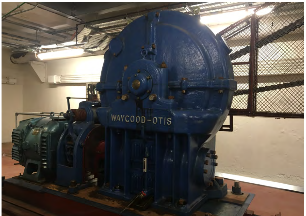
These original motors from the 1950's will form part of the permanent reminder of the engineering heritage of the tunnel on display.
