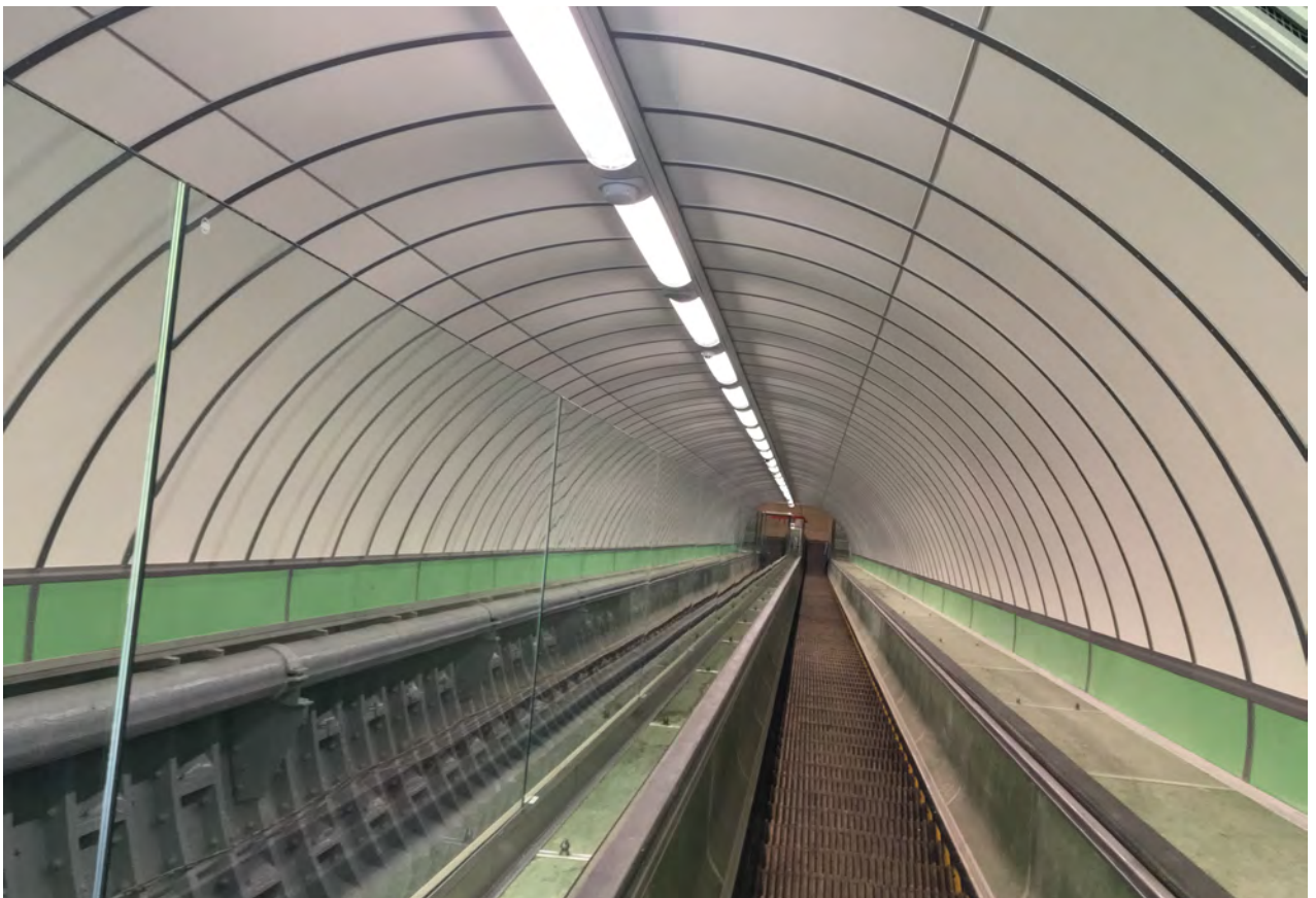
The inclined escalator shaft works have been completed with a glazed screen erected down the centre to provide a barrier to the new inclined lift.
