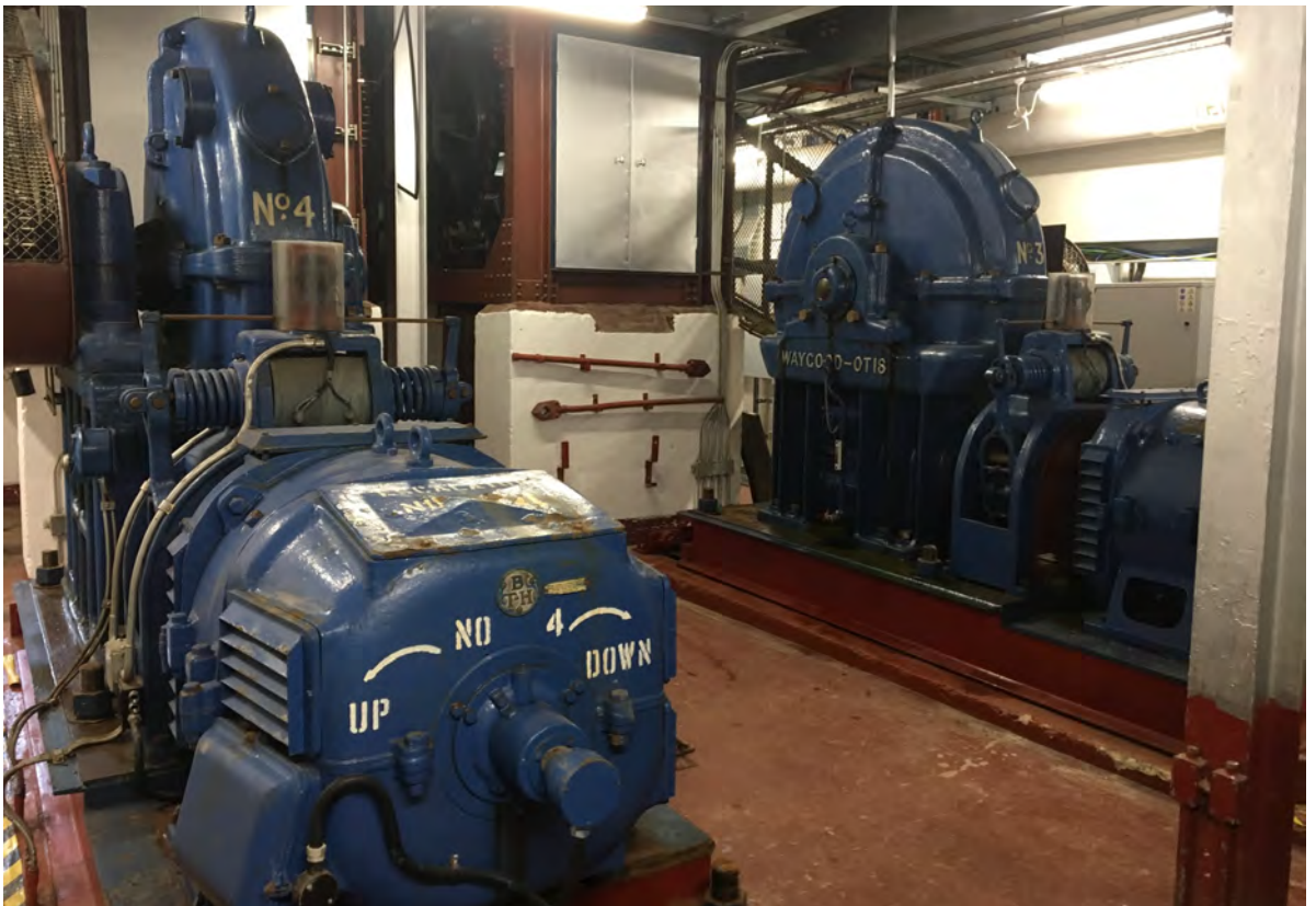
During the refurbishment the original 'Waygood-Otis' escalators motors have been under wraps. These have now been uncovered.
