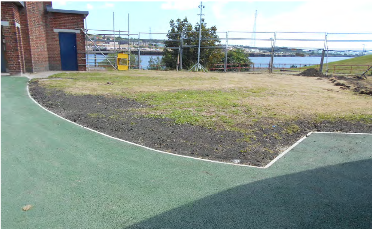
The landscaping and resurfacing works around the Jarrow rotunda building have been completed.
