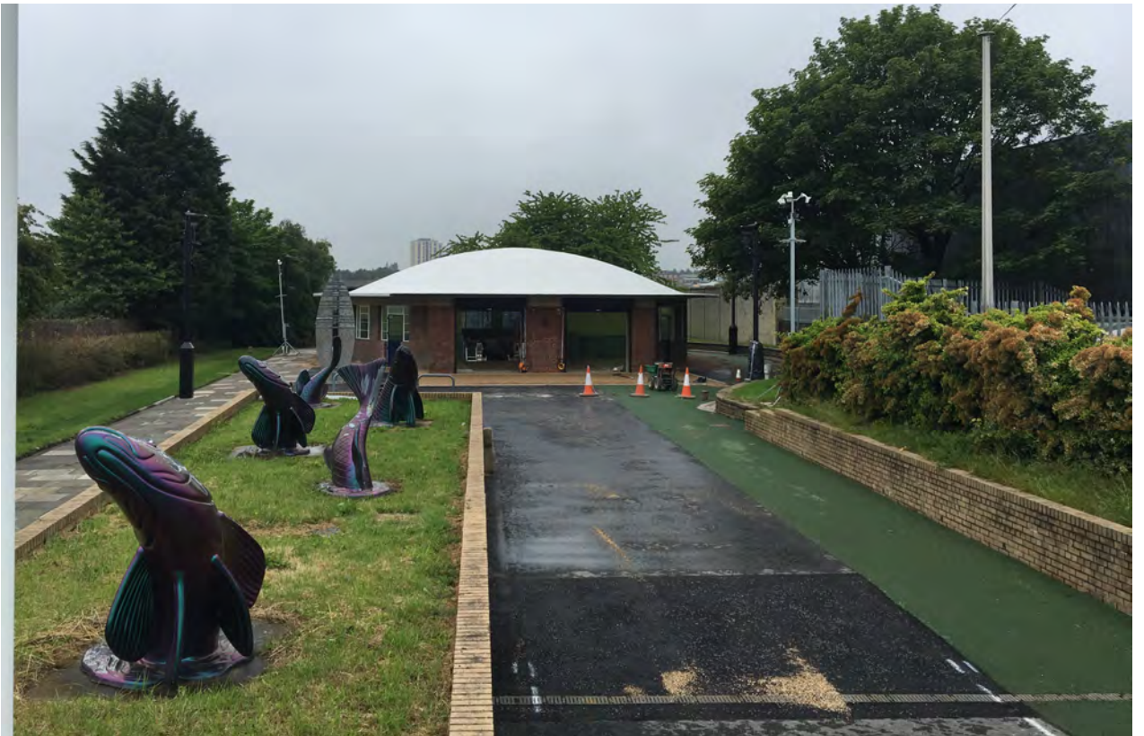
The new surfacing to the approaches to the Howdon rotunda building and the landscaping works have been finished. Only the road markings remain to be completed.
