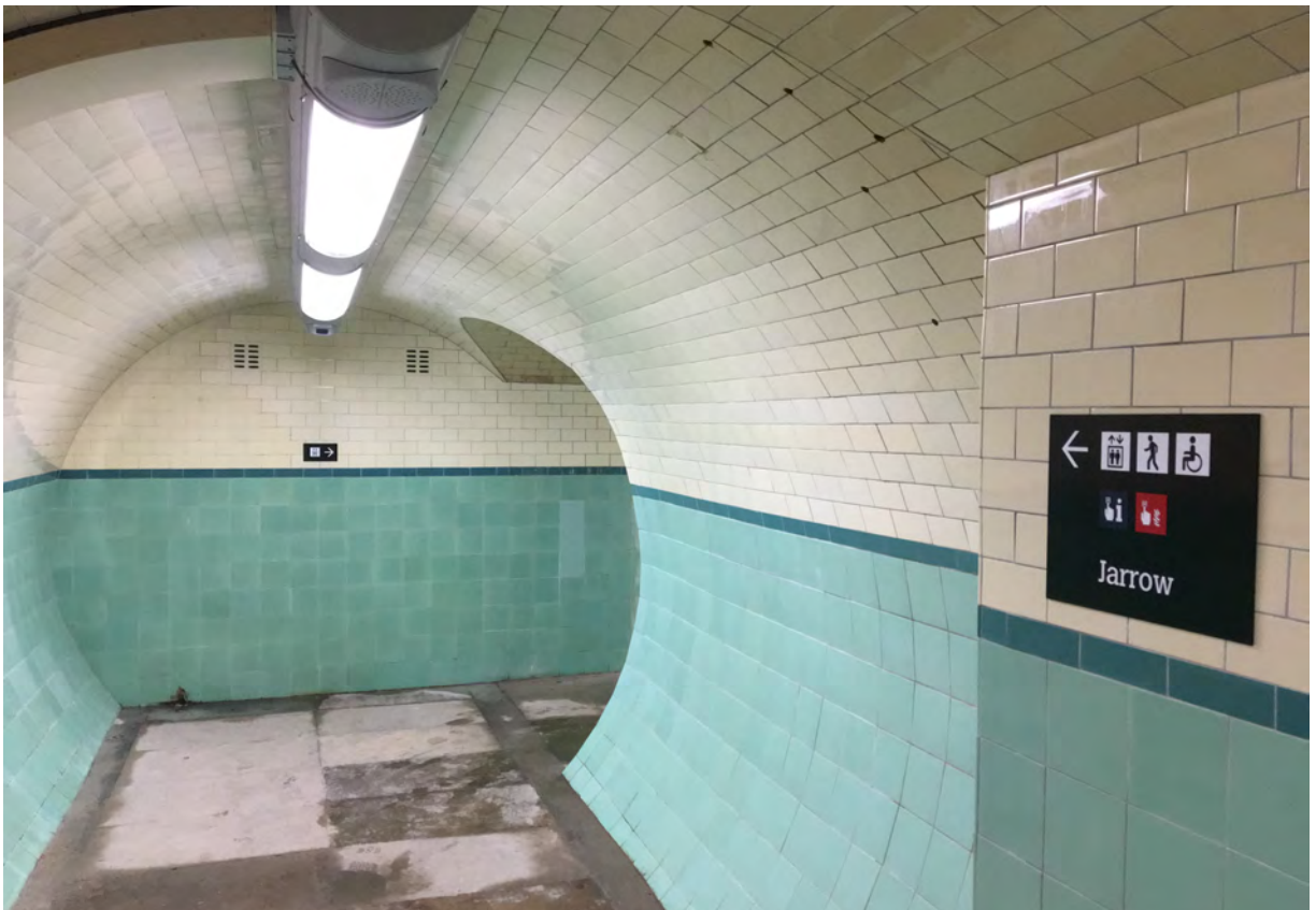
The link tunnels to the vertical lifts are complete and the direction signs have now been erected.
