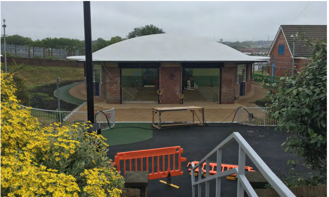
The new surfacing to the approaches to the Jarrow rotunda building and the landscaping works have been finished. Only the road markings remain to be completed.
